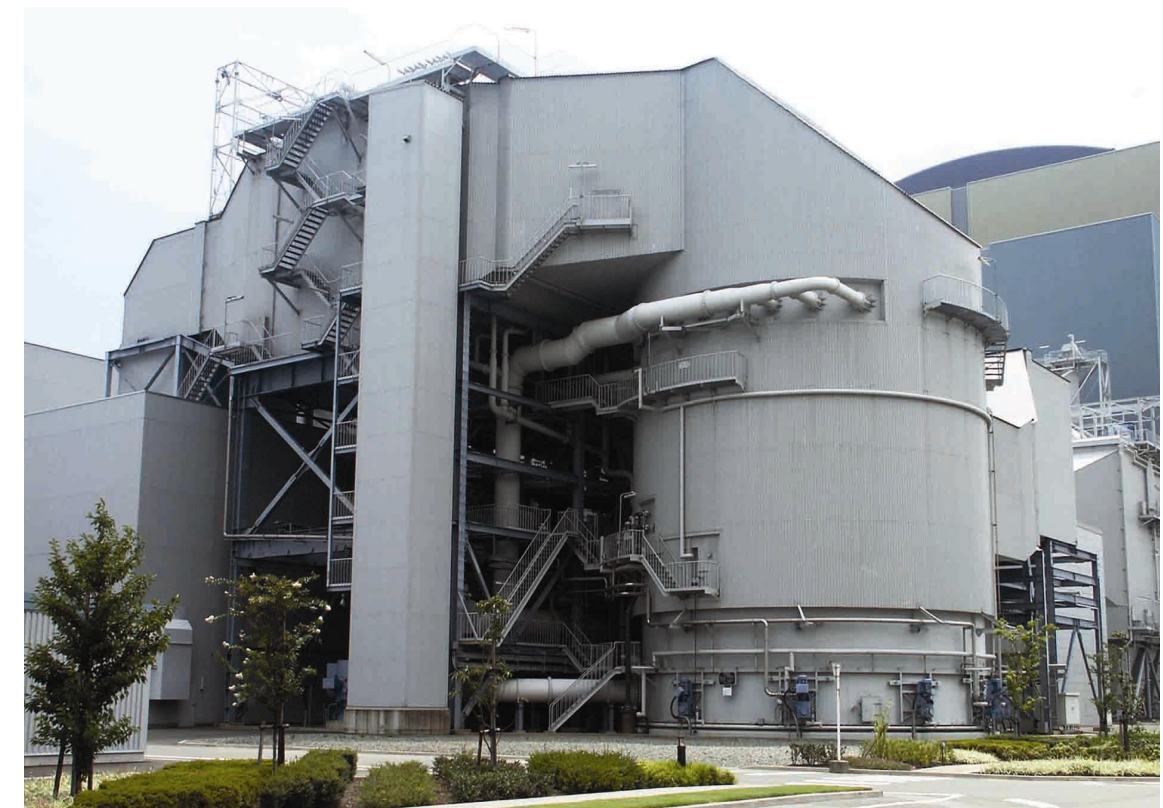
1050MW AQCS at J-Power-Tachibanawan
